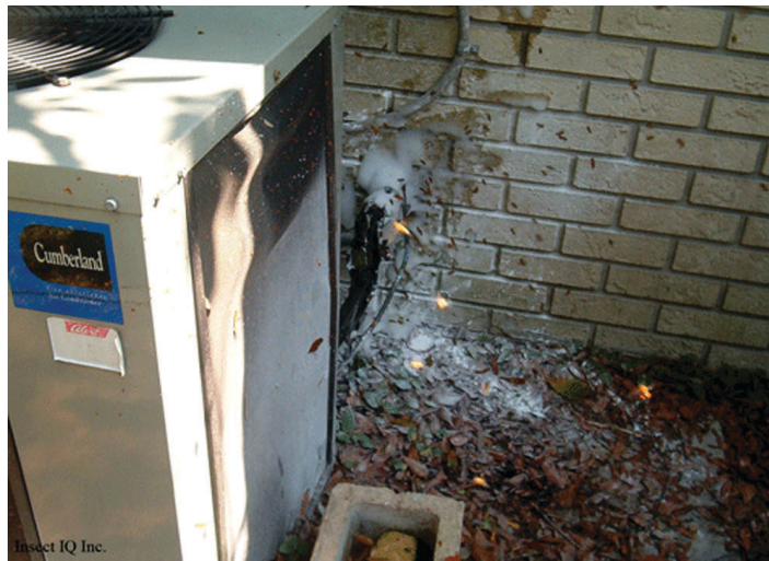
Figure 22. Colony eradicated from wall behind AC unit. Foam was used to block the entrance.
