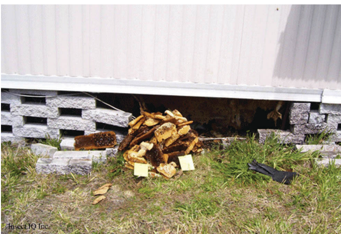
Figure 18. Colony removed from the underside of building. Credits: AllFloridaBeeRemoval.com
