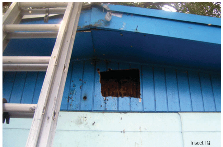
Figure 15. Colony removed from inside a wall under the eave of building.
