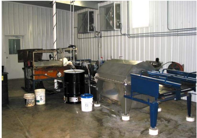
A commercial honey processing facility.
