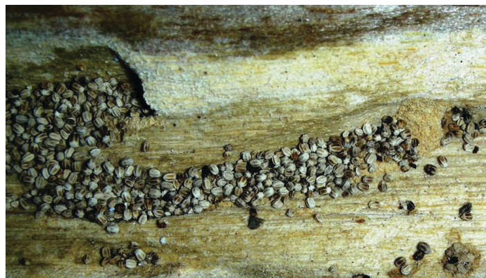
Figure 8. The galleries of drywood termites are excavated through the wood regardless of grain. The walls of the galleries are clean with dry loose fecal pellets.
